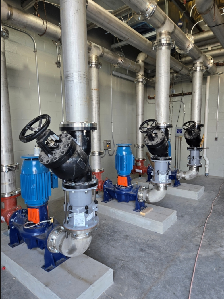
Boiler Pumps and Piping
