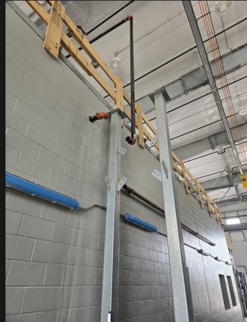
Example of minor conflicts between piping and structural supports
