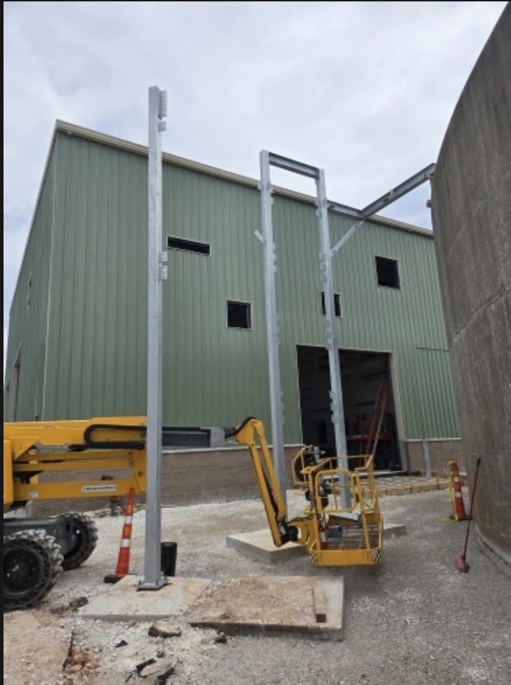
Exterior supports for drag link conveyance system from dryer facility to silo
