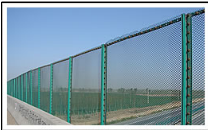
Figure 2-4: Expanded Metal Fence
