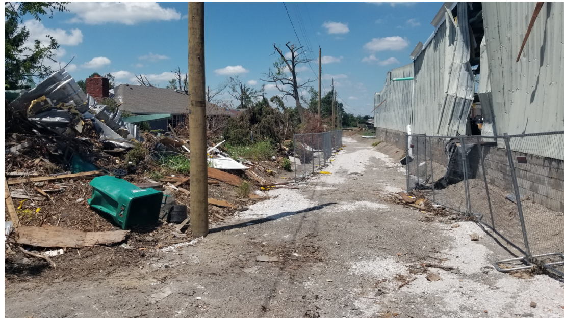
Photo: Looking down the proposed alignment of the proposed sewer improvement project from Chateau Dr. to Innisfree assisted living. This was one of the most severely impacted areas of town. The design is being re-evaluated after the damages due to the loss of trees, buildings, and relocation of power poles.
