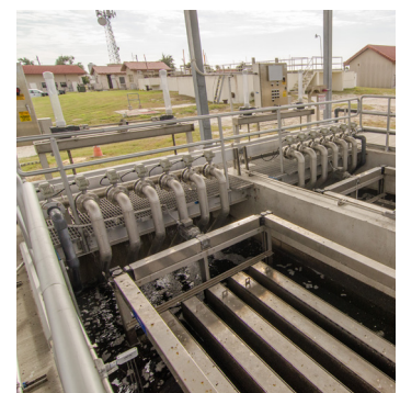
Corpus Christi Whitecap WWTP Disk Filters (designed by Jason Cocklin)
